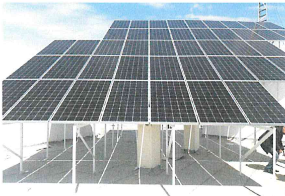
PV Cells - Emirati RC Hospital
